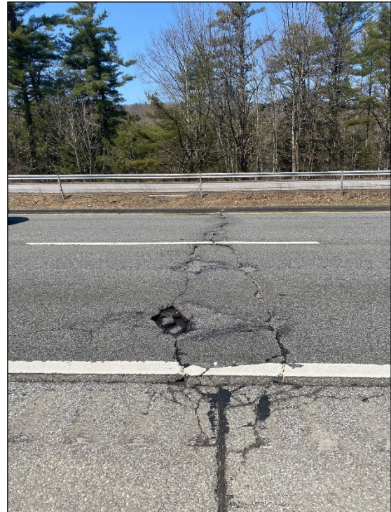
A portion of I-295 in Cumberland County showing extensive cracks and spalling.
